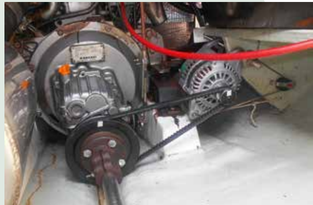
This installation ran successfully on a 42ft catamaran with twin 34hp Yanmar engines. Unfortunately sideways pull on the propshaft disturbed the engine mounts, so it is now being rebuilt with a strut from the engine to the alternator. See lifepart2.info/equipment/prop-shaft-driven-alternator
