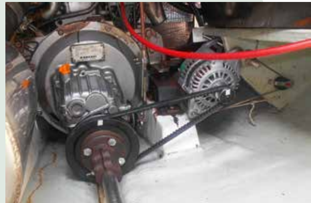
This installation ran successfully on a 42ft catamaran with twin 34hp Yanmar engines. Unfortunately sideways pull on the propshaft disturbed the engine mounts, so it is now being rebuilt with a strut from the engine to the alternator. See lifepart2.info/equipment/prop-shaft-driven-alternator
